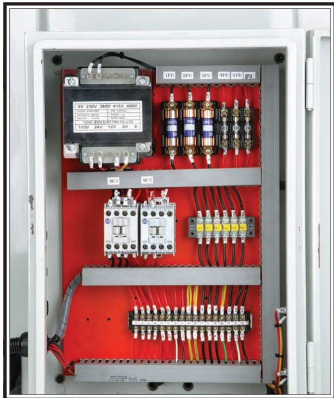
Figure 72. SB1025 Electrical box.
